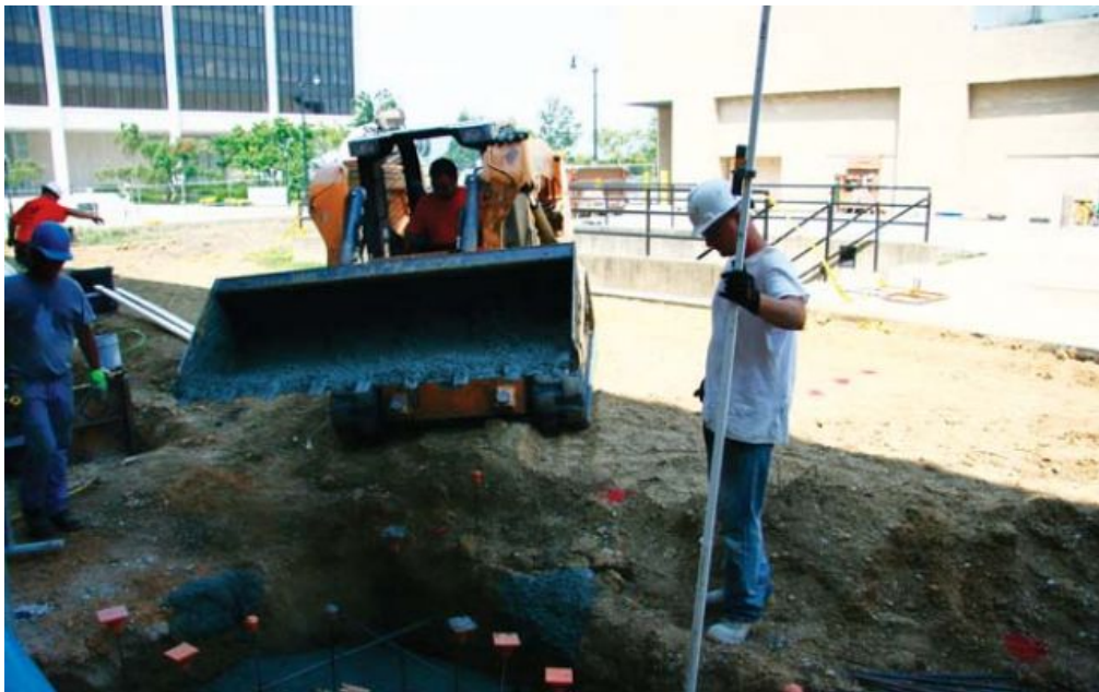
Construction is underway on the PCCC's new outdoor plaza. PHOTO BY PATRICK YEAGLE
